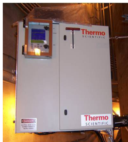
Figure 3: View of the Alpha test installation at a coal-fired plant
